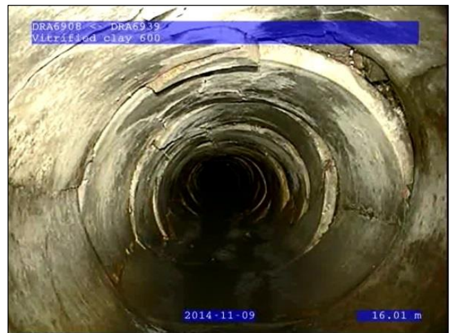
Condition 5 – Very Poor
