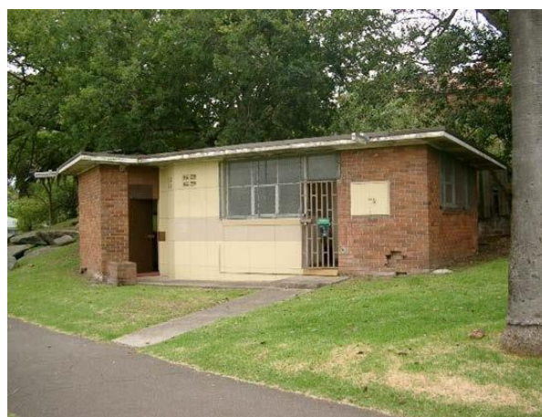
Condition 5 – Very Poor
