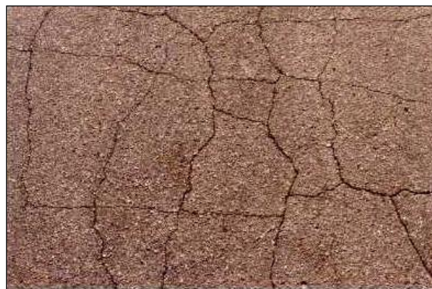
Condition 5 – Very Poor
